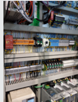
THE DESIGN & MANUFACTURING OF THE ELECTRICAL PANELS ARE MADE ACCORDING TO THE CANADIAN REGULATION (CSA)
